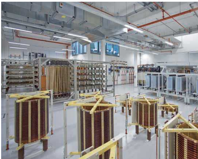
Fig. 22: Resistance and inductance on the high- and low-voltage side of the testing transformer
