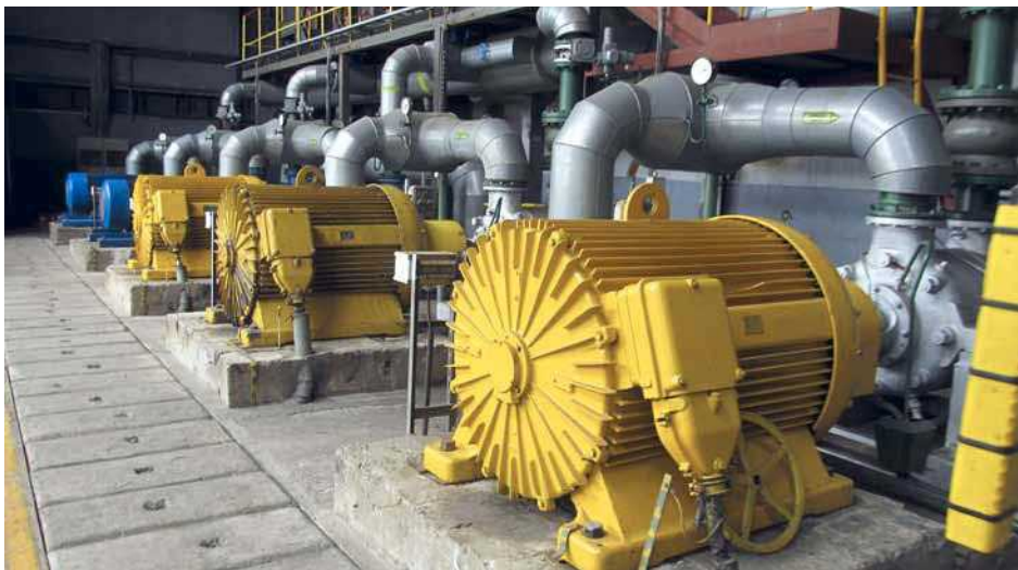
Fig. 2: Electric motors with high power induce surge voltages due to high switch-on currents
